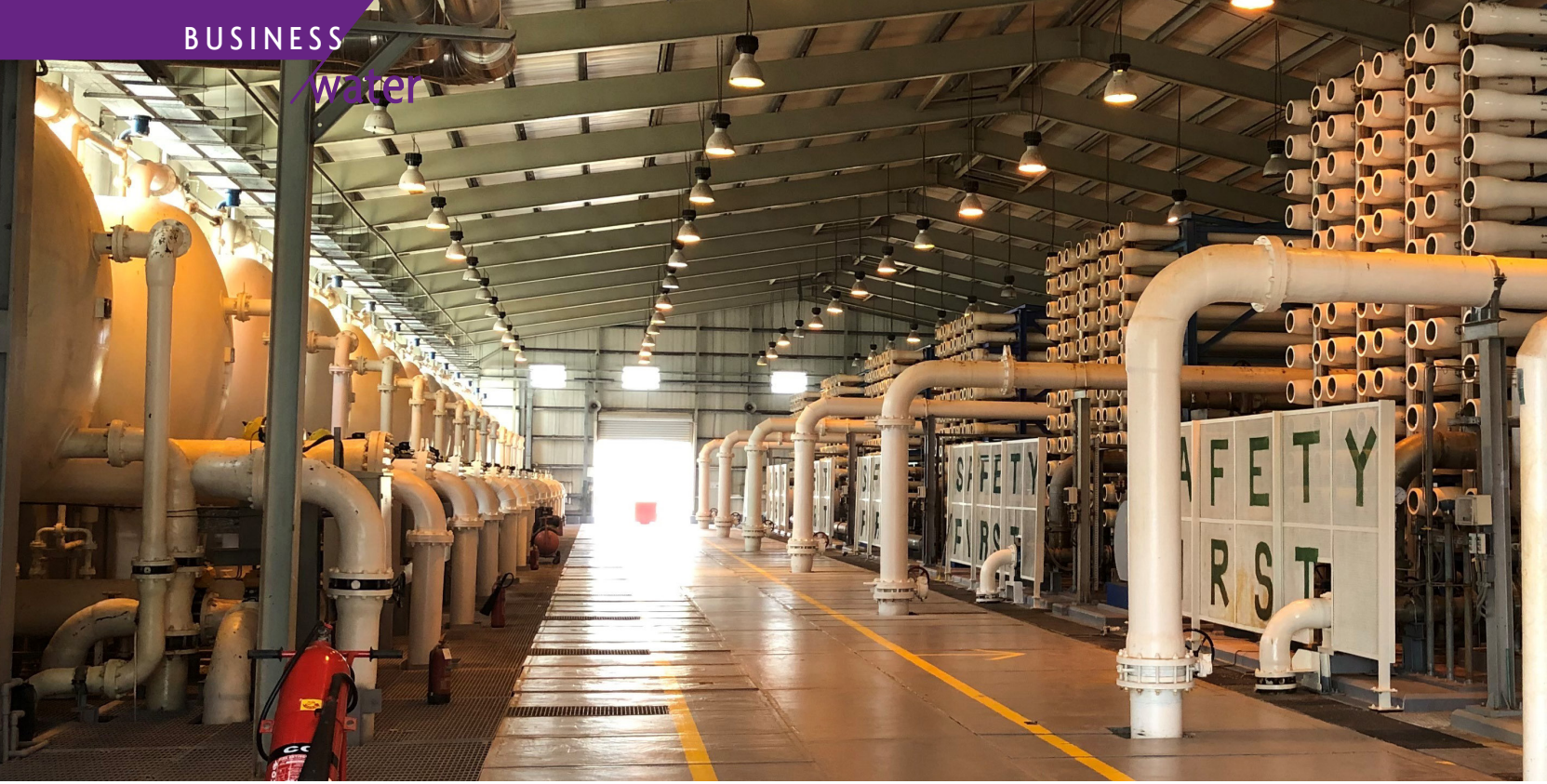
Interior of the desalination plant at the international airport in Jeddah (Saudi Arabia).
